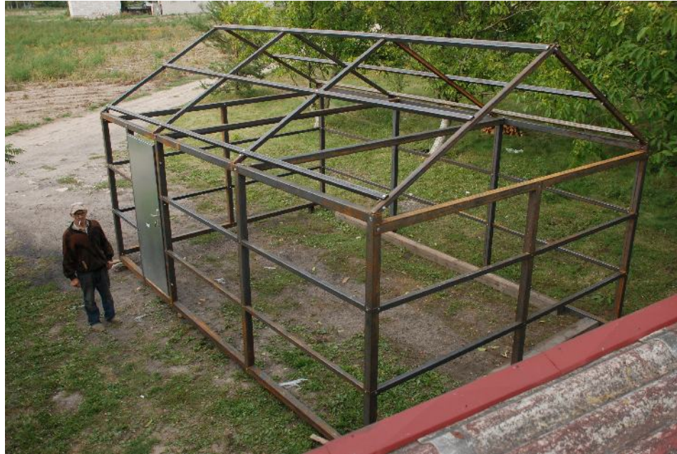
A metal structure built by Stanisław Adamski and Adam Pesta in Kurówko, 2015
